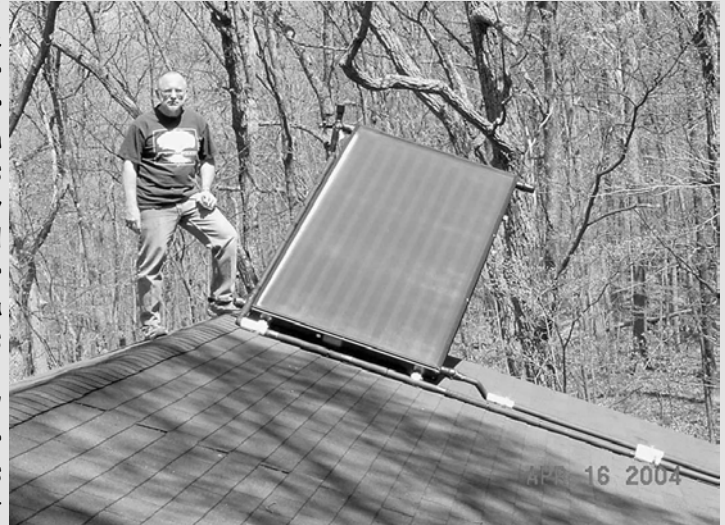
Figure 6.4: Steve Boyce on his roof with his solar water heater collector, Andy McDonald
