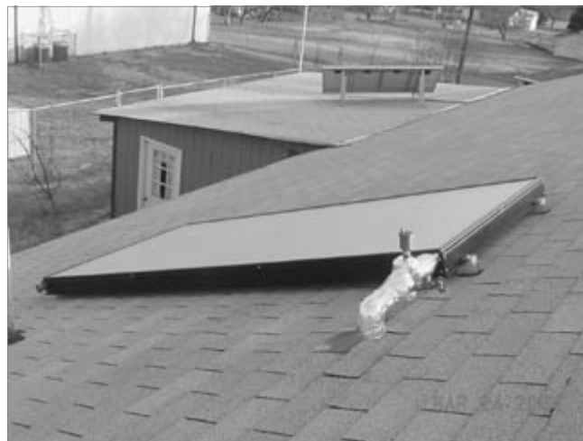
Figure 6.1: A solar collector on the roof of ASPI's Small Town Demonstration Center in Mt. Vernon, Kentucky, Andy McDonald
